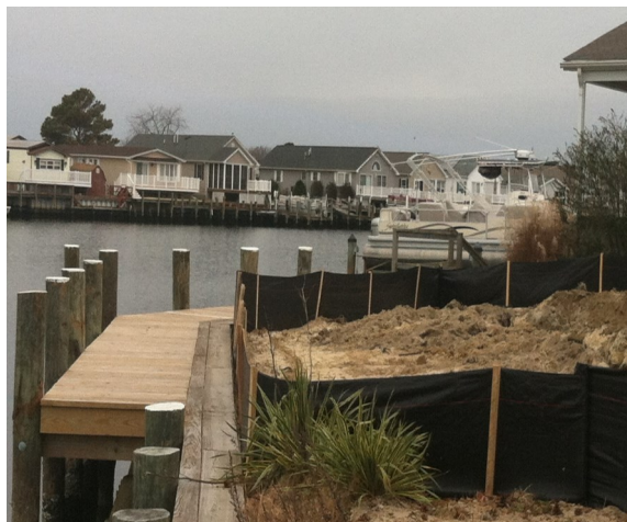
Single family home construction within Critical Area setback with erosion and sediment control Ocean City, Maryland
