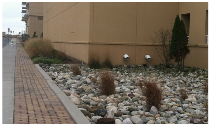
Porous paver sidewalk extensions adjacent to SWM treatment facility, Ocean City, Maryland
