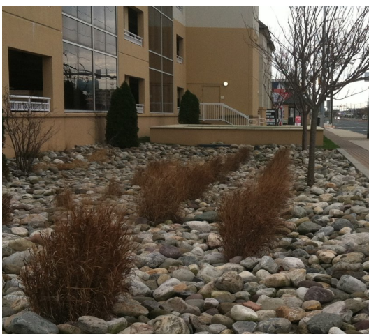
Landscaped SWM treatment facility Ocean City, Maryland
